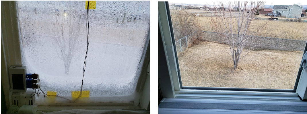
Figure 12. Left: Condensation and ice buildup on interior surface of Helena, MT field site (double-pane windows, vinyl frame). Right: Same window location after replacement with the thin triple pane window (fiberglass frame). Both photos are taken in March 2021 at a similar time of day, but outdoor and indoor conditions vary between photos.
