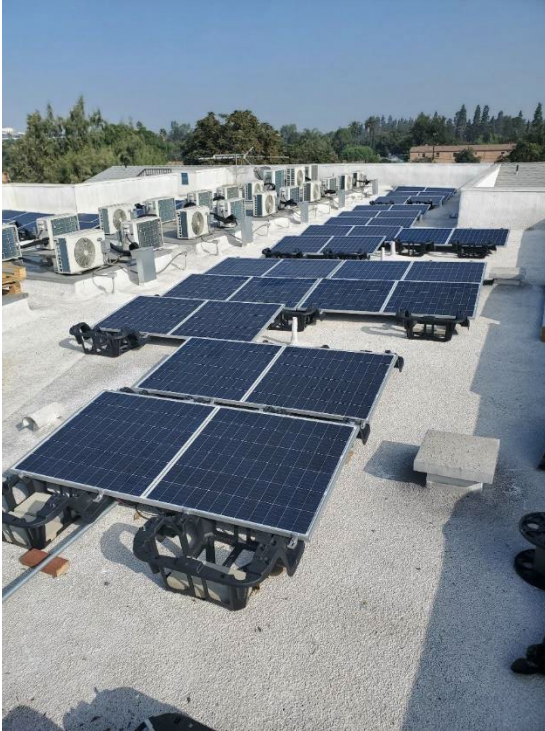
Figure 3: Bifacial PV Installation. Source: EPRI, 2021.
