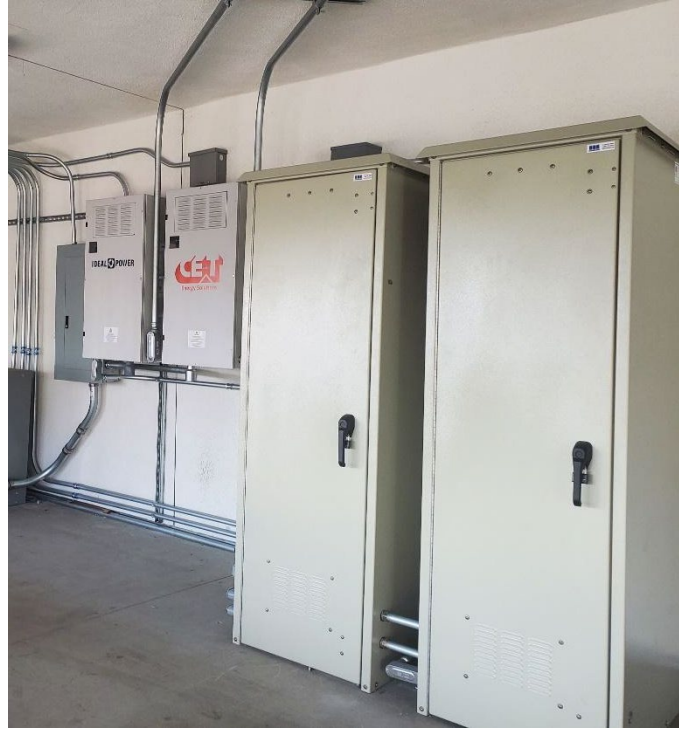
Figure 4: Installed Inverters (Left) and Batteries (Right). Source: EPRI, 2021.
