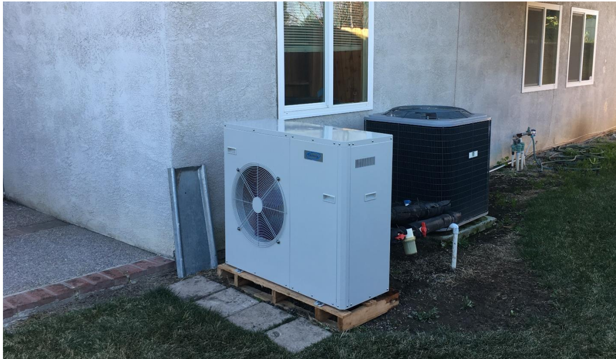
Figure 7. Installed variable capacity AWHP.
