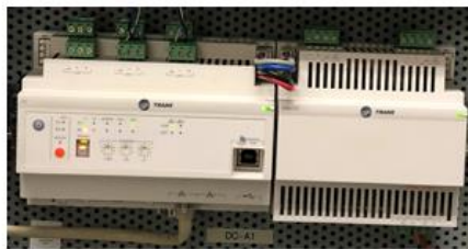
Building Control System
