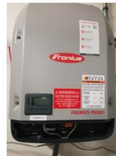
Solar PV Inverter
