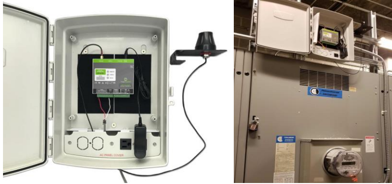
Figure 3. Cellular real-time monitoring equipment used for the pilot. A complete real-time kit is shown on the left prior to installation, and a picture of a completed installation is shown on the right.
