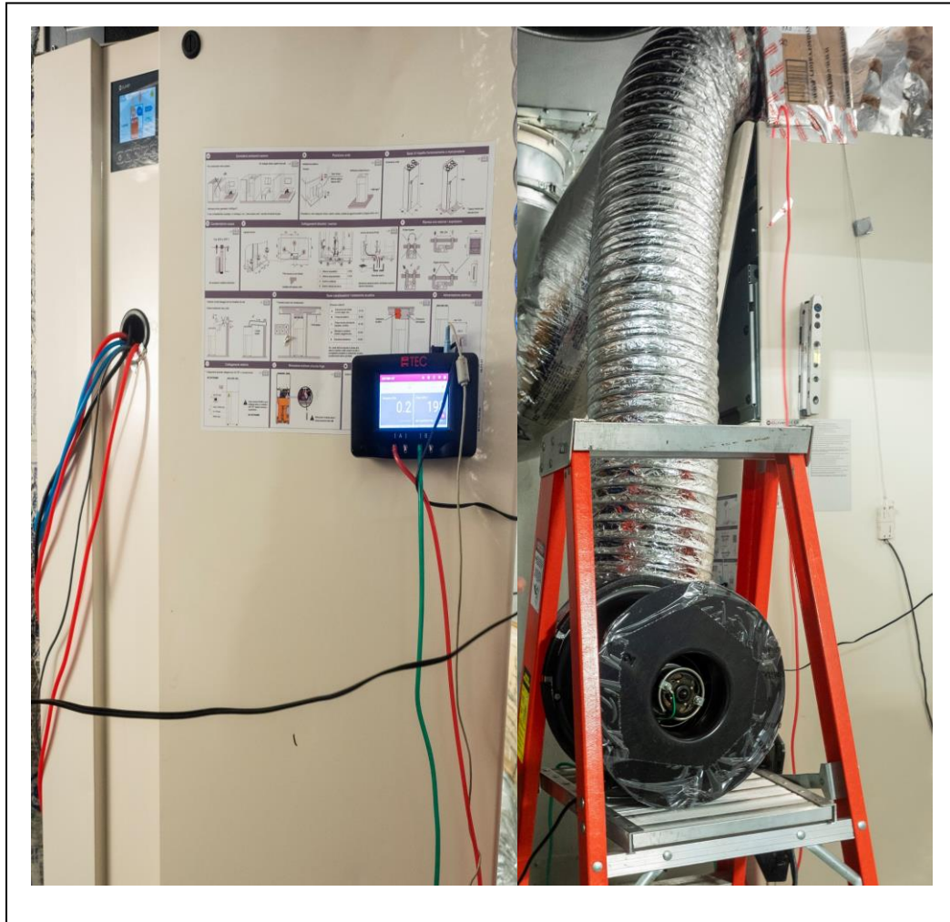
Figure 3: Calibrated fan setup as a powered flow hood to measure return air flow from conditioned space
