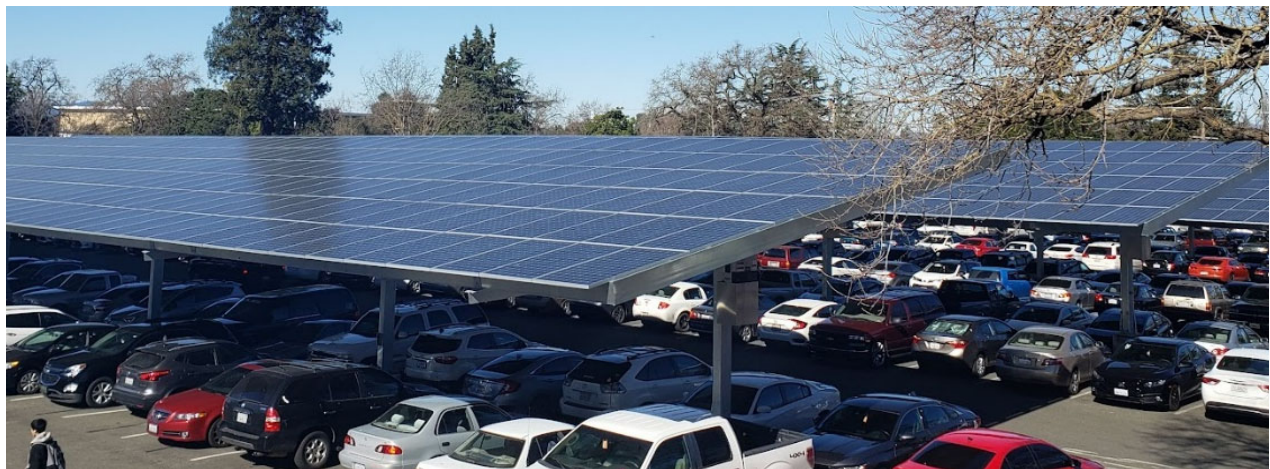
Figure 3. Carport PV Panels at the Bech Hall Parking Lot. Source: Santa Rosa Junior College
