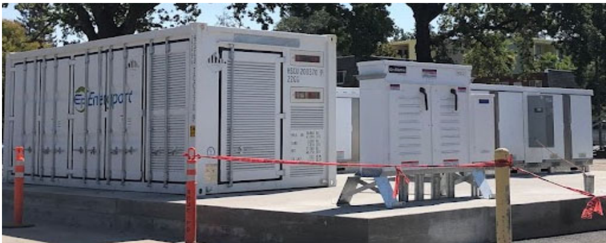
Figure 4. Energport Battery System and GoElectric Inverter at Emeritus Hall. Source: Santa Rosa Junior College
