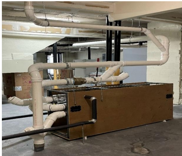
Figure 6. Installed Level-2 Drain Water Heat Recovery System
