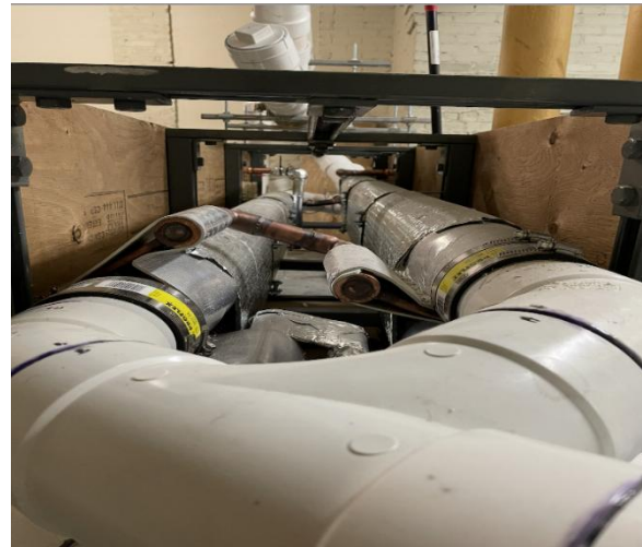
Figure 7. Interior View of Level-2 Drain Water Heat Recovery System
