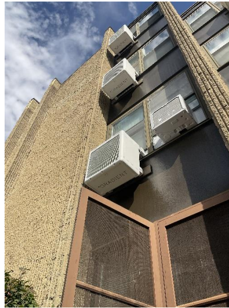
Figure 9. Exterior View of Installed Saddle Style Heat Pumps
