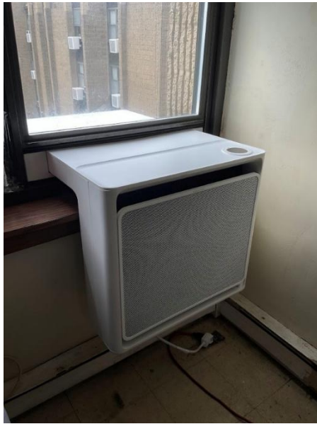
Figure 8. Interior View of Installed Saddle Style Heat Pump
