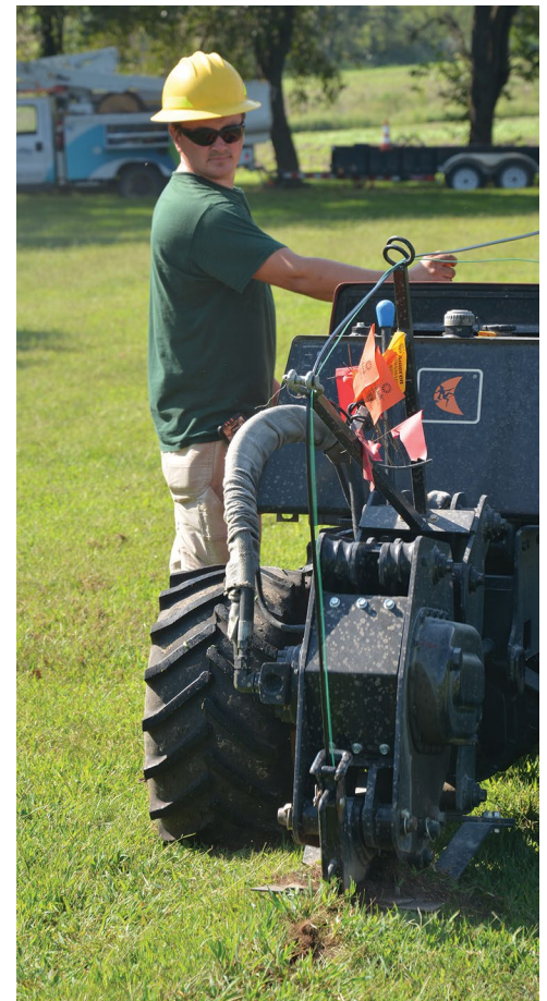
AJ Hagedorn, a lineman at Co-Mo Electric's subsidiary Co-Mo Connect, installs fiber along the right-of-way to deliver gigabit broadband-enabled energy efficiency to its members. Source: Co-Mo.
