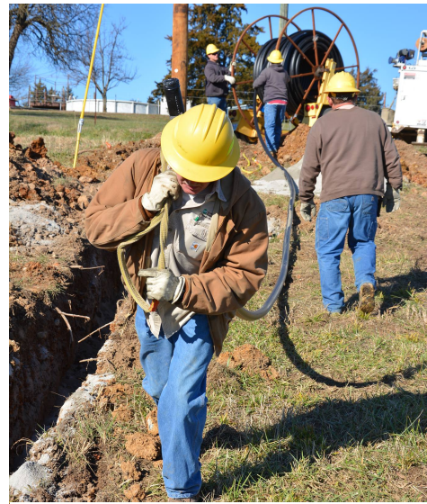
A lineman at Co-Mo Electric's subsidiary Co-Mo Connect installs fiber along the right-of-way (above) to deliver gigabit broadband-enabled energy efficiency to its members. Source: Co-Mo 2018b.
