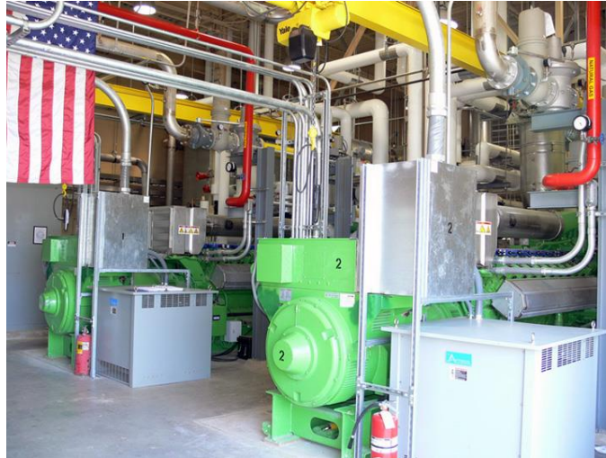
Figure A1. Cogeneration facility at BCUA's Little Ferry Water Pollution Control Facility. Source: BCUA 2015.
