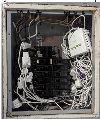
Figure 5. Energy meter installed on an electrical panel
