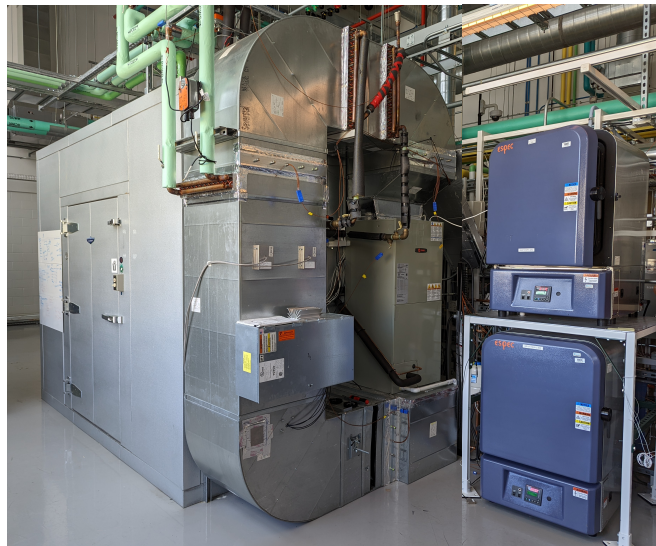
Figure 3. HVAC hardware-in-the-loop system: Outdoor unit sits inside the chamber, air handler is connected to duct loop, and thermostat sits inside lower blue environmental chamber
