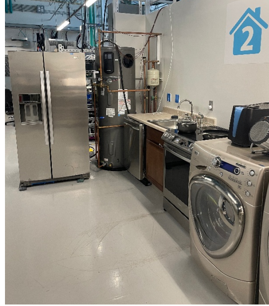
Figure 2. Laboratory setup refrigerator, heat pump water heater, dishwasher, range, washer, and dryer.
