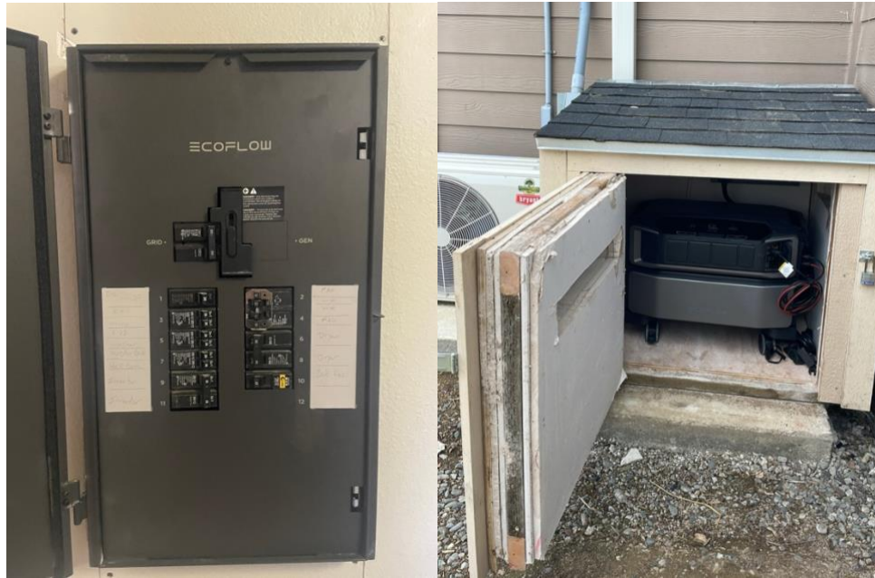
Figure 7. Design configuration #1 - 240V, 1 ph., 100A service, installed new smart home panel, and plug-in batteries (inverter and batteries installed in an enclosure)
