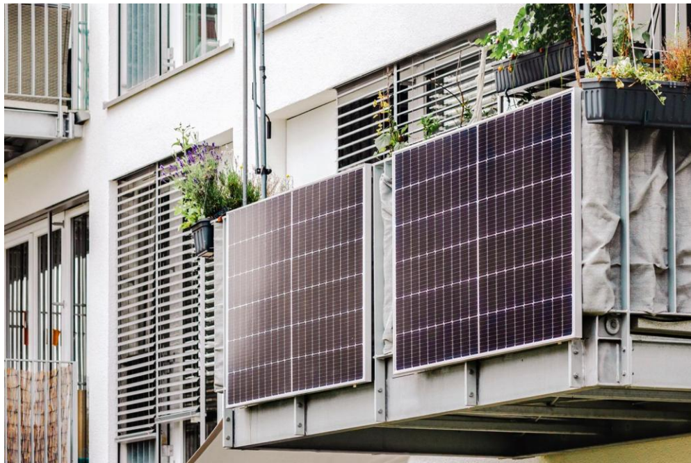
Figure 12. Example of a balcony solar system installed on an apartment. Source: Canary Media
