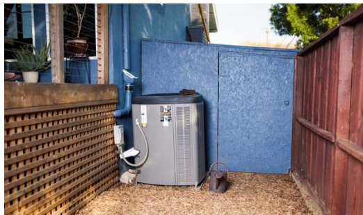
Figure 5. Outdoor unit, Central HP Image Source: California HP Partnership
