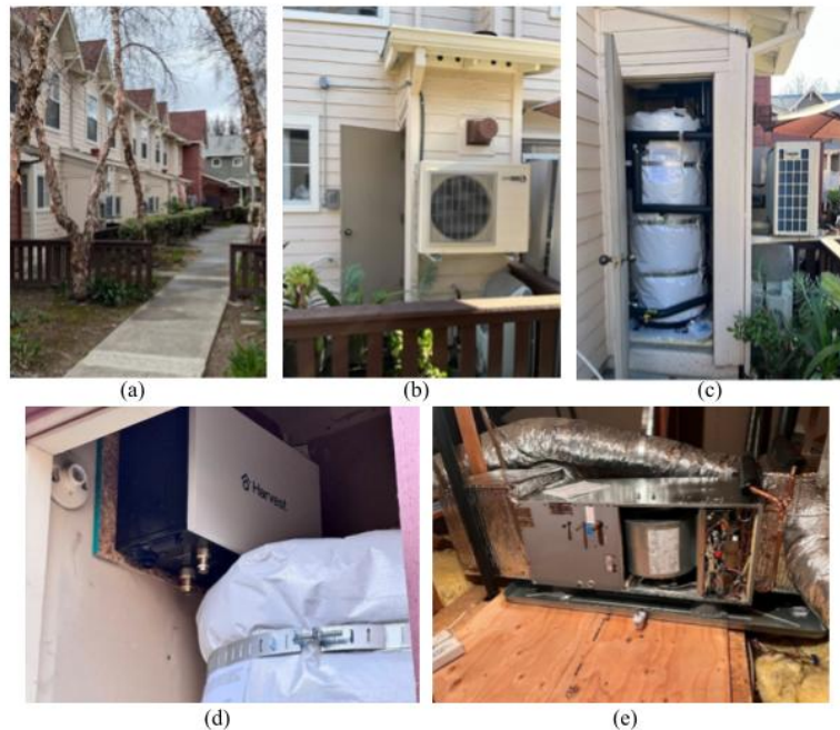
Figure 2: (a) Heat Pump Condensers in Back Alley; (b) Heat Pump Condenser on Water Heater Closet; (c) Thermal Energy Storage Tank in Water Heater Closet; (d) Harvest Pod in Water Heater Closet; (e) Air Handler in Attic
