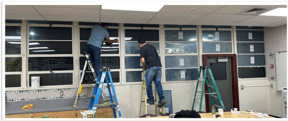
Figure 4. CSW Retrofit at Site 1: Junior High. Photos provided by vendor. 2025.
