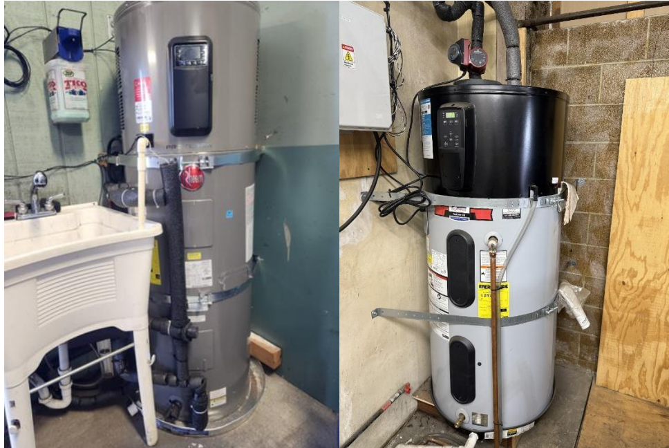
Figure 1. Installed 120V heat pump water heaters at site 2 (left) and site 3 (right). Source: EPRI.
