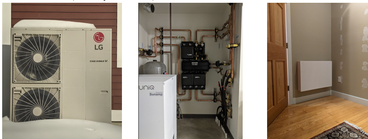
Figure 5: Massachusetts pilot installation. Left: LG Therma V R32 AHP outdoor unit. Center: Sunamp UniQ PCM TES unit (white cabinet), Caleffi pump stations and balance-of-plant components. Right: JAGA Briza ductless hydronic fan coil unit.
