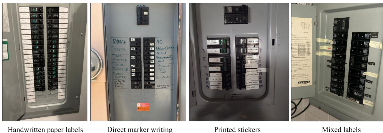
Figure 4: Representative examples of individual breaker labeling formats observed in residential panels.
