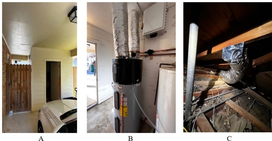
Figure 10. Replacement of a conventional water heater in a carport shed (A) with a 120 V HPWH (B) dual-ducted to the attic (C). Source: Pilet (2024).
