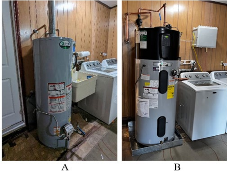
Figure 6. Replacement of a conventional water heater (A) with a 120 V HPWH (B) installed in an attached garage. Source: Pilet (2024).
