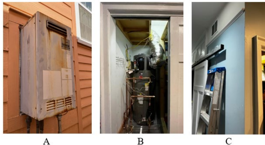
Figure 2. Replacement of an outdoor tankless water heater (A) with a 120 V HPWH (B) installed in a closet with a flex duct and grille retrofit (C). Source: Pilet (2022).
