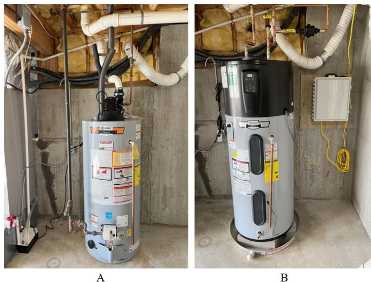
Figure 4. Replacement of a conventional water heater (A) with a 120 V HPWH (B) installed in a basement. Source: Guerrieri (2025).
