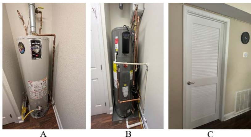
Figure 1. Replacement of a conventional water heater (A) with a 120 V HPWH (B) installed in a utility room with a louvered door (C). Source: Pilet (2024).
