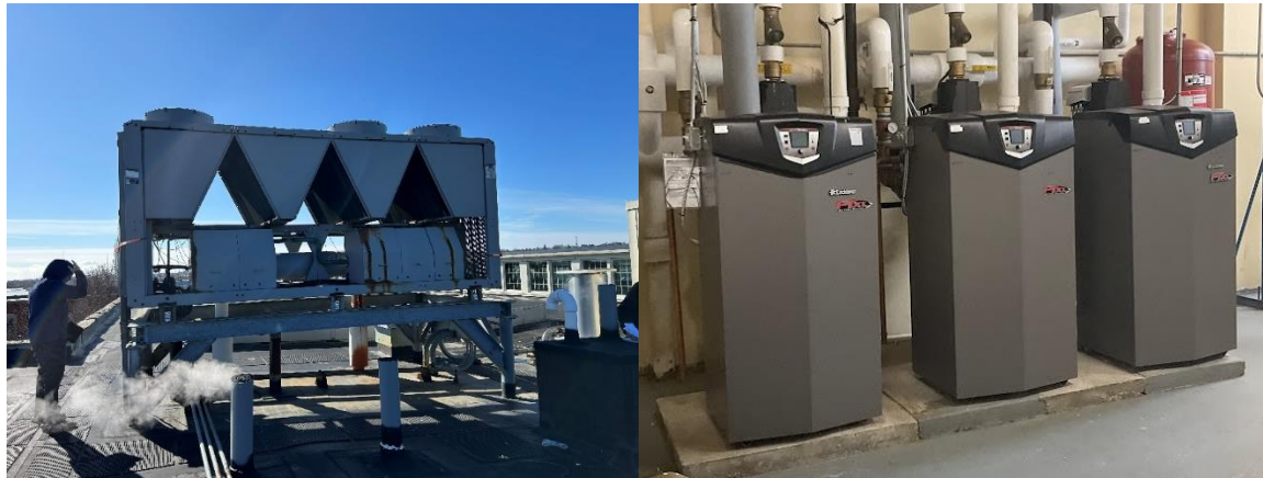
Figure 1. End of life Carrier 30RBA 120-ton air cooled chiller (left), and three Lochinvar model FTX850N boiler plant (right)
