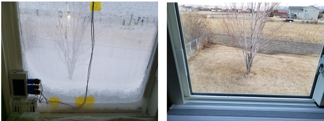
Figure 7. Helena, MT, field study, March 2021. Left: double-pane, vinyl framed window shows condensation and ice buildup. Right: Same location after replacing double-pane with thin triple-pane fiberglass-framed window, shows zero condensation and ice buildup.
