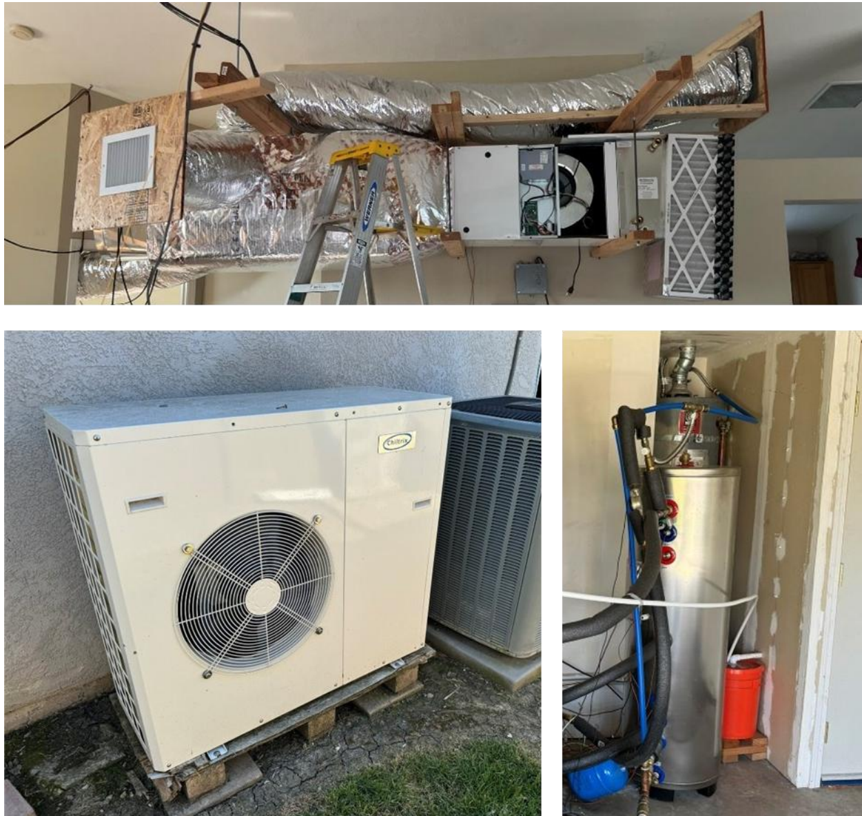
Figure 3. Three of four primary components of the Three-Function AWHP system are pictured including a ducted fan coil unit (top photo) outdoor AWHP (bottom left), and a DHW tank (silver water tank in the bottom right).
