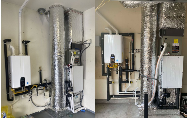
Figure 3. Final installed system at Site 1 (left) and Site 7 (right).
