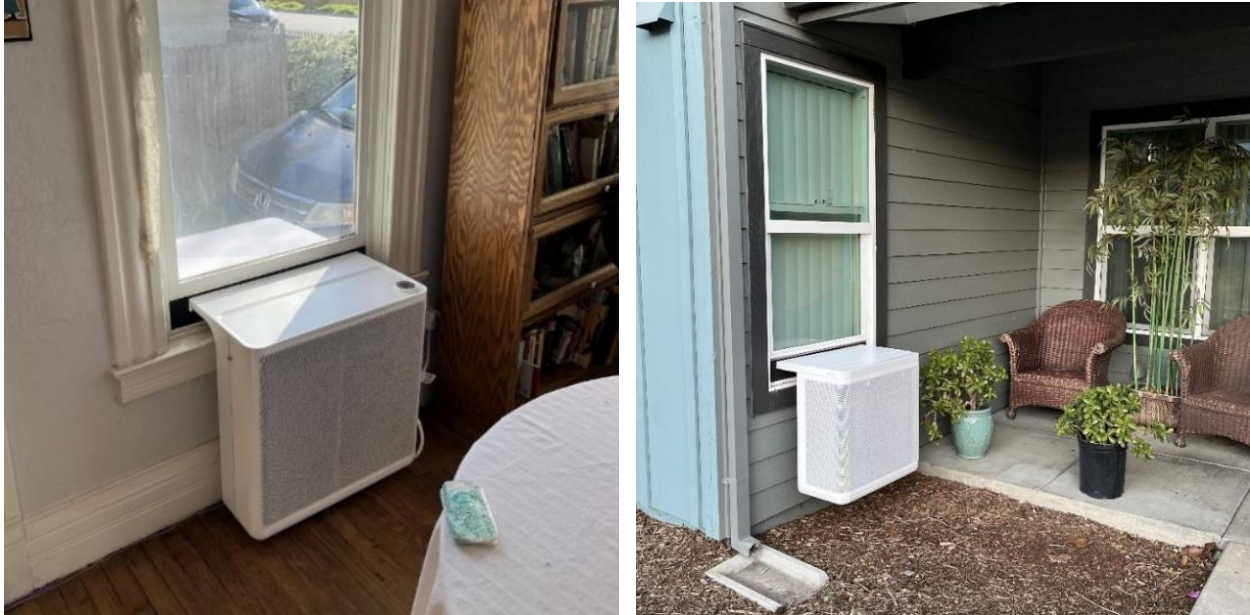
Figure 1: Gradient heat pump indoor unit (left) and outdoor compressor unit (right) installed at demonstration sites.
