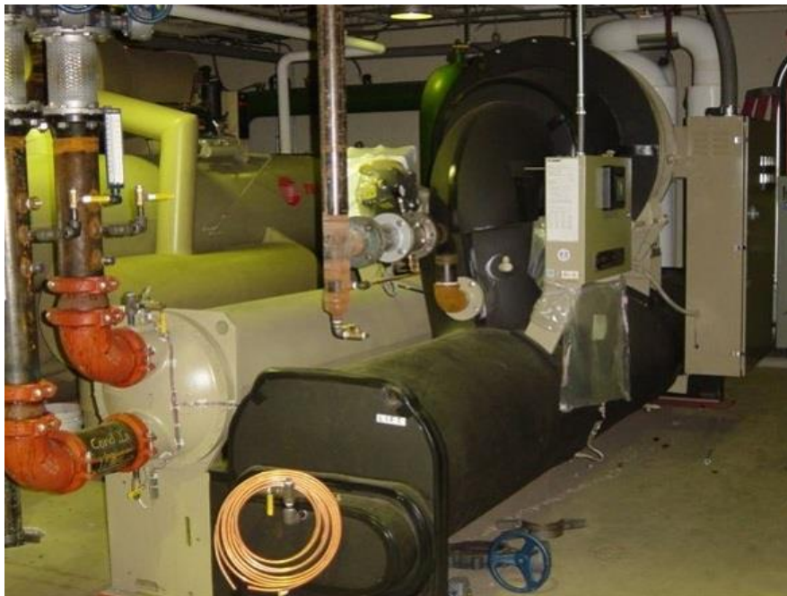
Figure 8. Example of a 250-ton heat recovery chiller used for facility hot water and HVAC applications (Source: Alabama Power)
