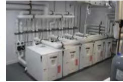
Ground-source heat pump system
