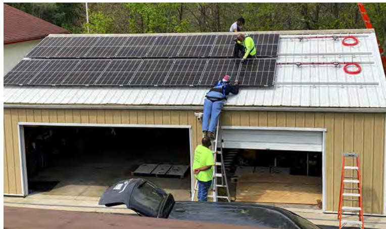
Workers finish installing a 6-kW solar array on a storage garage at Crowley Engineering's Indiana headquarters. Source: Crowley Engineering LLC ( crowleyengineering.com ).
