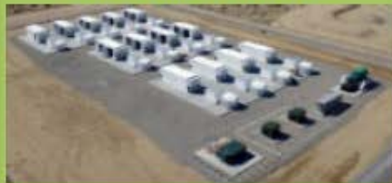
Battery energy storage
