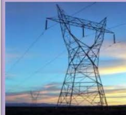
Increased capacity on external transmission
