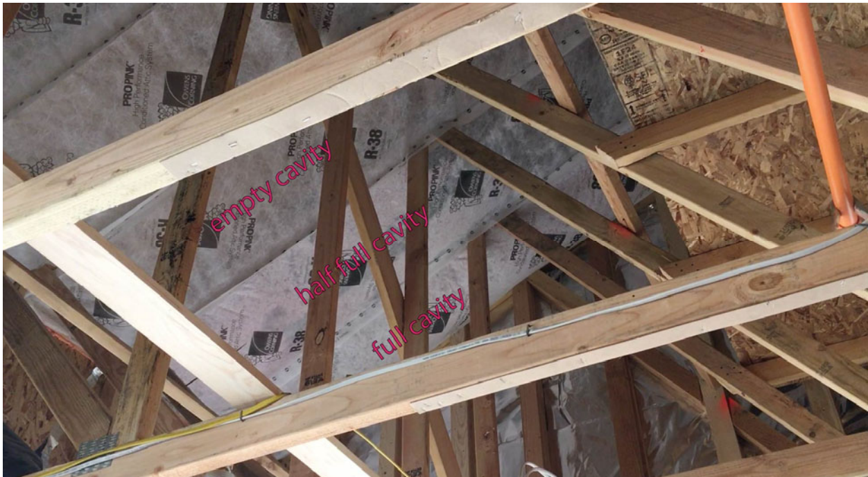
Figure 1. Installing insulation under roof deck with boxed netting solution. Source: Can Anbarlilar, PG&E.
