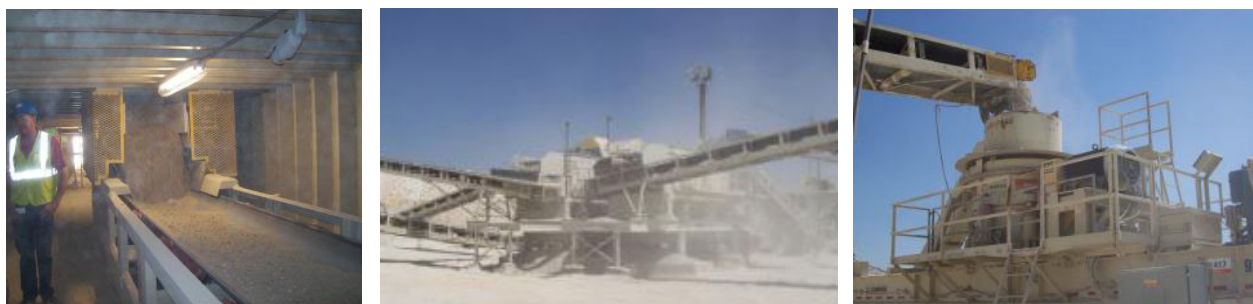
Figure 4. Photos left to right: feeder conveyor, cone crusher, and close-up of cone crusher.
