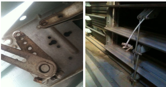
Figure 11. Common Economizer Failures
