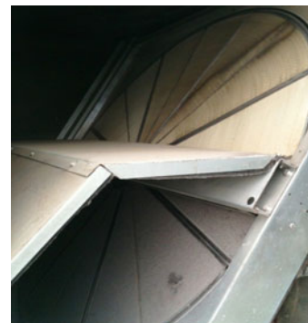
Figure 12. Broken belt on ERV
