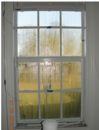
Figure 6. Unvented tight house north-facing window condensation January 23, 2013.
