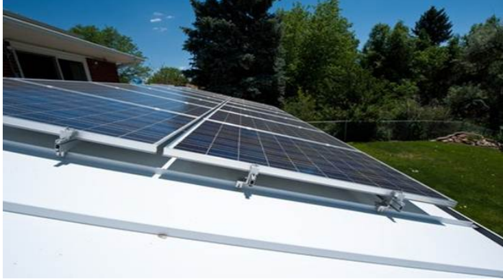
Figure 1. Roof Mounted Arrays and Wire Management
