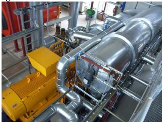
Figure 1: Installed ORC Power Generator
