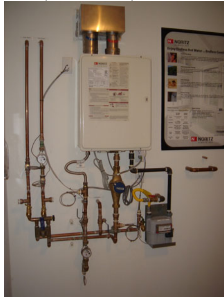
Figure 6. Tankless On-Demand Water Heater With Instrumentation Including Flow Meters, Gas Meters, and Thermocouples
