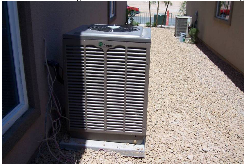
Figure 3. The Freus Evaporative Cooled Condensing Unit at the ZEH and the Conventional Condensing Unit for the Baseline House in the Background
