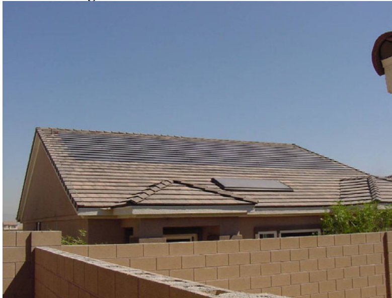
Figure 5. Photograph Taken From the Neighboring Yard of the South Facing ZEH Roof With the Roof Integrated Photovoltaic Panels and Solar Water Heater
