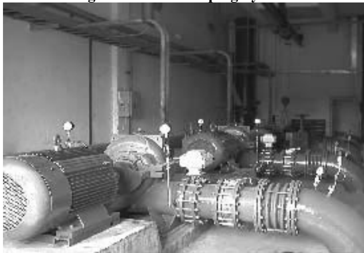
Figure 4. New Pumping Systems
