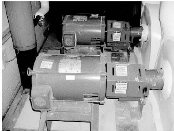
Figure 5. Circulation Pumps at a 50,000 SF Elementary School. The Big Pump (10 Hp.) is for Cooling, the Little Pump (3 Hp.) is for Heating.
